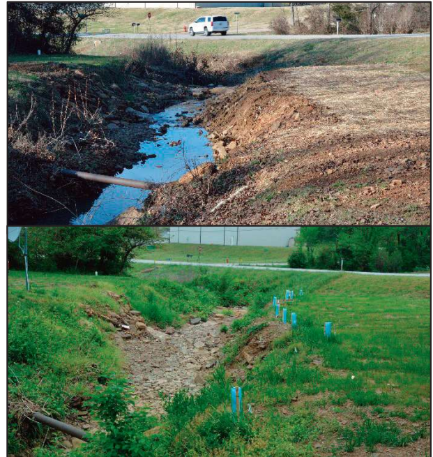
This riparian area was cleared by a municipality in order for a new water line to be installed (top). Tree seedlings and grass seed were planted during a restoration effort (bottom). (Photos by Bryant Baker)
